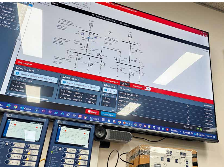
Image 3: Ronald Jogaib uses RelaySimTest to demonstrate to his customers the correct behavior of SEL protective devices in case of a fault.
