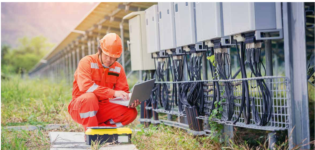
Technician testing a photovoltaic installation
