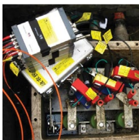
Example of using an HFCT in a cross bonding box
