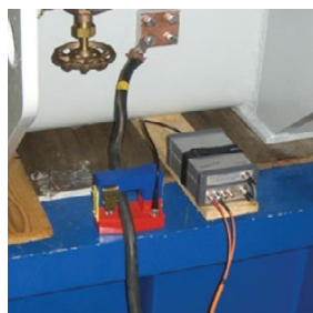
Example of HFCT grounding cable at a power transformer
