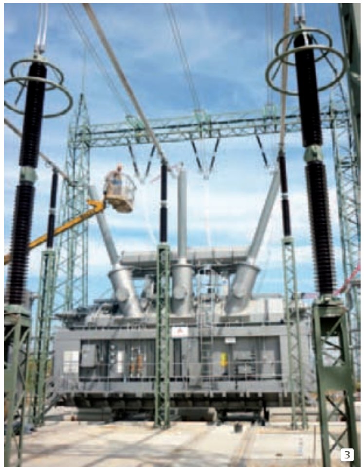
1 Primary testing device for generating up to 2,000 A with connection cables to provide a primary supply. 2 Current transformer testing with the CT Analyzer on a current transformer in the bushing of a 30 kV E-reactor. 3 Current transformer testing with the CT Analyzer on a current transformer in the high-voltage bushing of a 380 kV power transformer.
