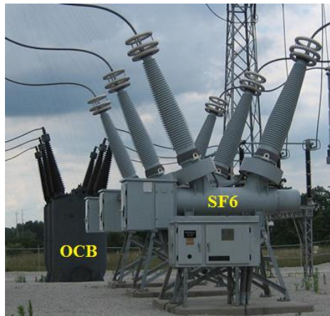
Figure 1 - Bulk OCB vs. Dead Tank SF6
