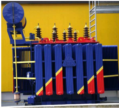
Figure 2: 6,5 MVA, 47 kV/27,2 kV power transformer
