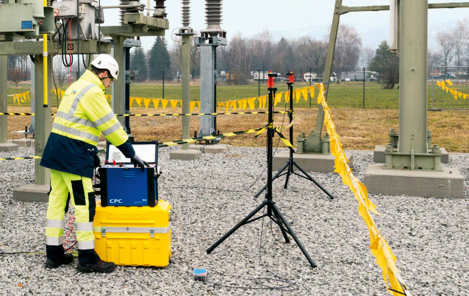
SAA2 in use onsite during transformer testing.
