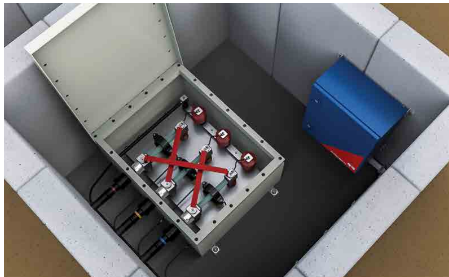
The cement boxes protect the HFCT sensors and data acquisition unit against ground water and dust.
