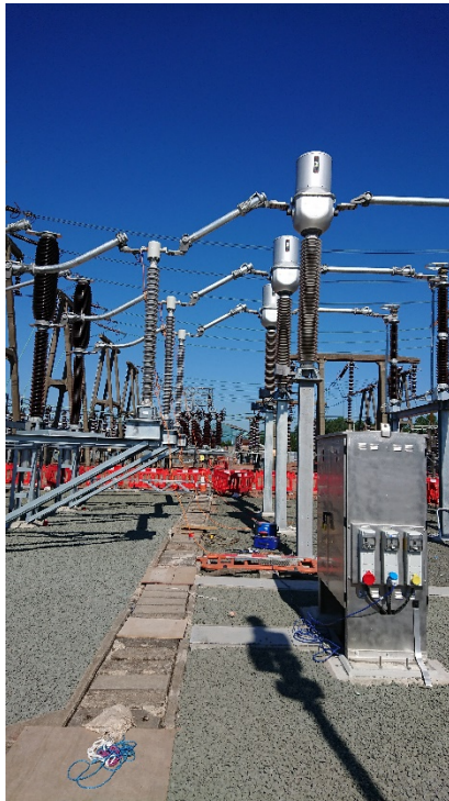
Fig. 7: Test with the CPC 100 in which the test current is driven by a conventional and a non-conventional transformer
