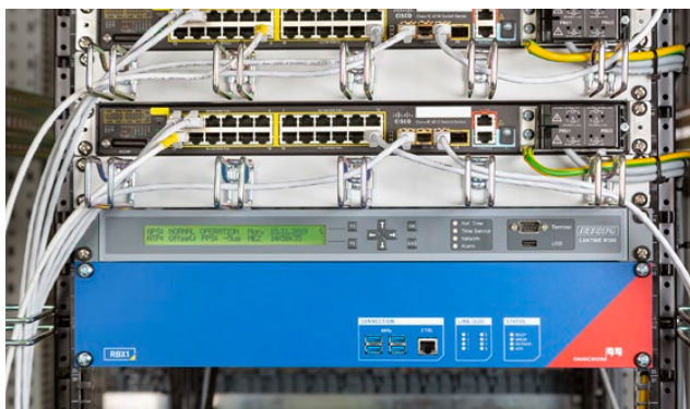
Figure 4: StationGuard installed in a greenfield 110kV substation, 2019
