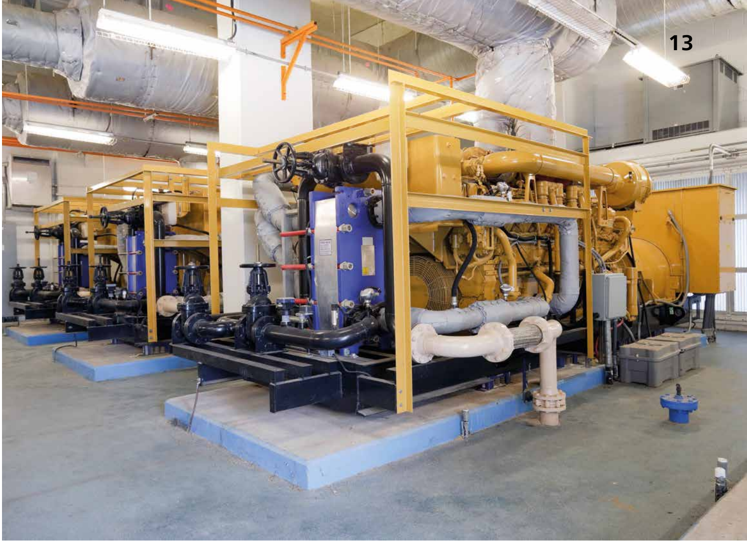
Customers of Gaal Umwelttechnik use medium-voltage generators on site to ensure a continuous, reliable power supply.
