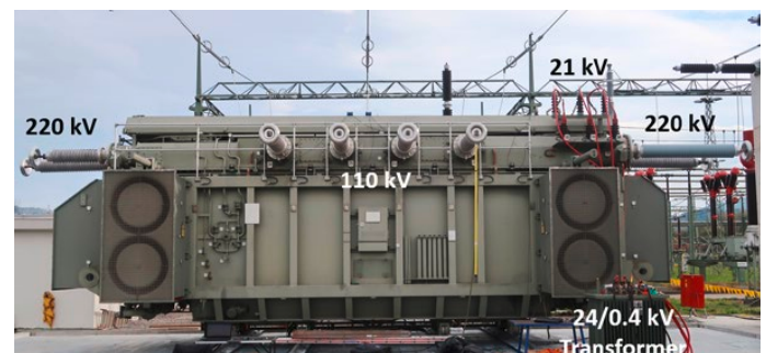
Figure 1 View of the 300 MVA Transformer
