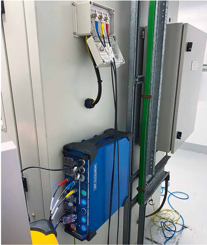
MONTESTO 200 can be easily mounted on the asset for continuous online PD monitoring for longer periods of time.
