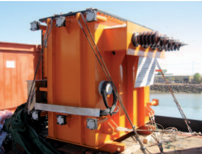
Singapore—Transformer damaged during shipping: DIRANA indicated that there was a water content of about 1 %. When this was combined with other electrical test results the transformer was found to be electrically sound. A significant amount of water had not spread to the paper insulation.
