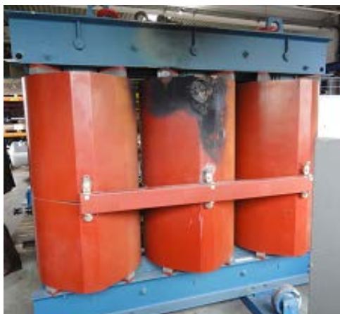
Figure 7. Breakdown fault on cast resin transformer
