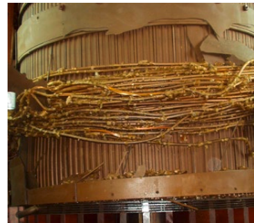
Collapsed tap winding
