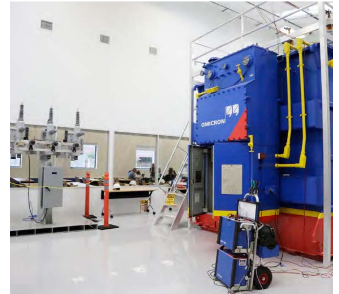
Indoor Substation for Hands-on Instruction
