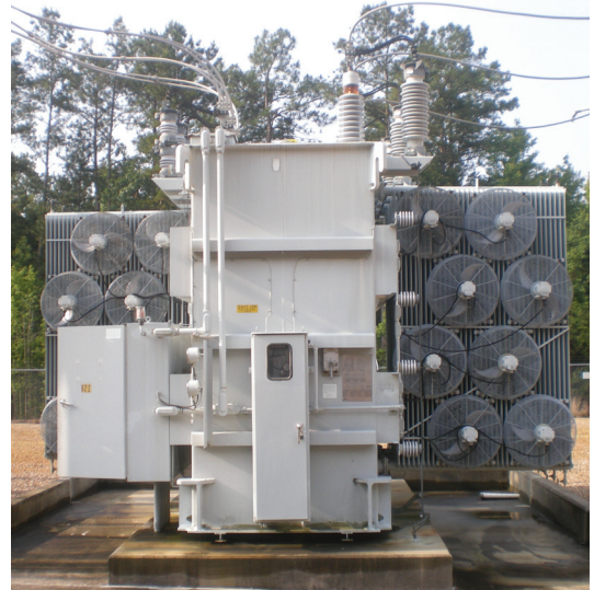
Bushings are a necessary component of a power transformer, but they are one of the transformer's main weaknesses.
