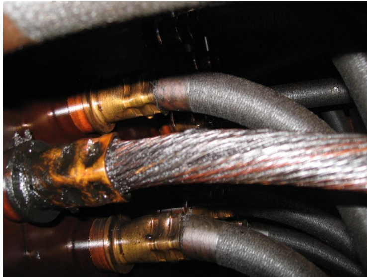
Figure 10 - Overheating of Connection #7
